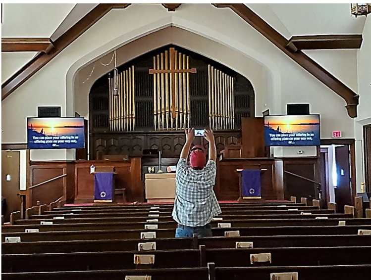
Nathan Hull checking out his work after the installation of the big screens.
